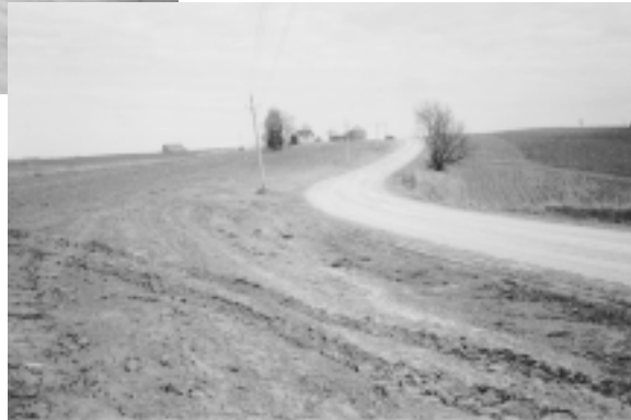
Above, beginning the work of eliminating a snow trap. At right, the left side of the road has been leveled off to eliminate a snow trap.
