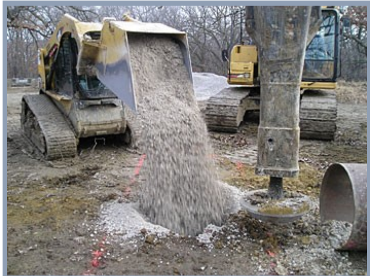
Placement of aggregate in drilled hole and special beveled tamper used for compaction (Geopier® system)
