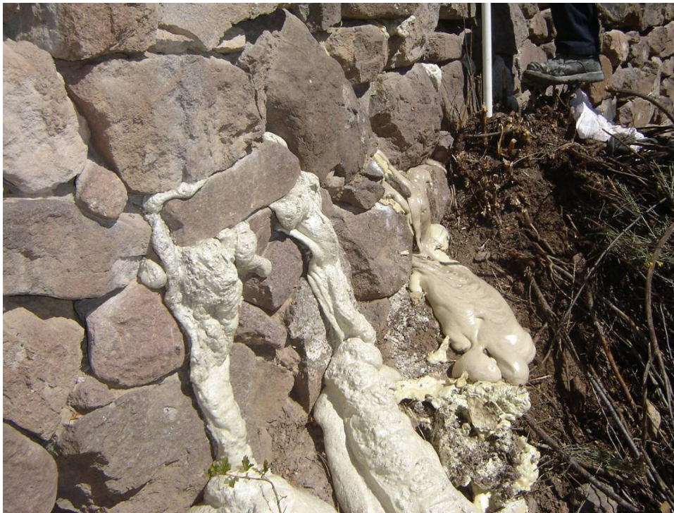
Figure 21. Photo. PUR that has foamed due to high moisture within the wall rock mass. This material can be readily peeled off the rock face and bagged for disposal.
