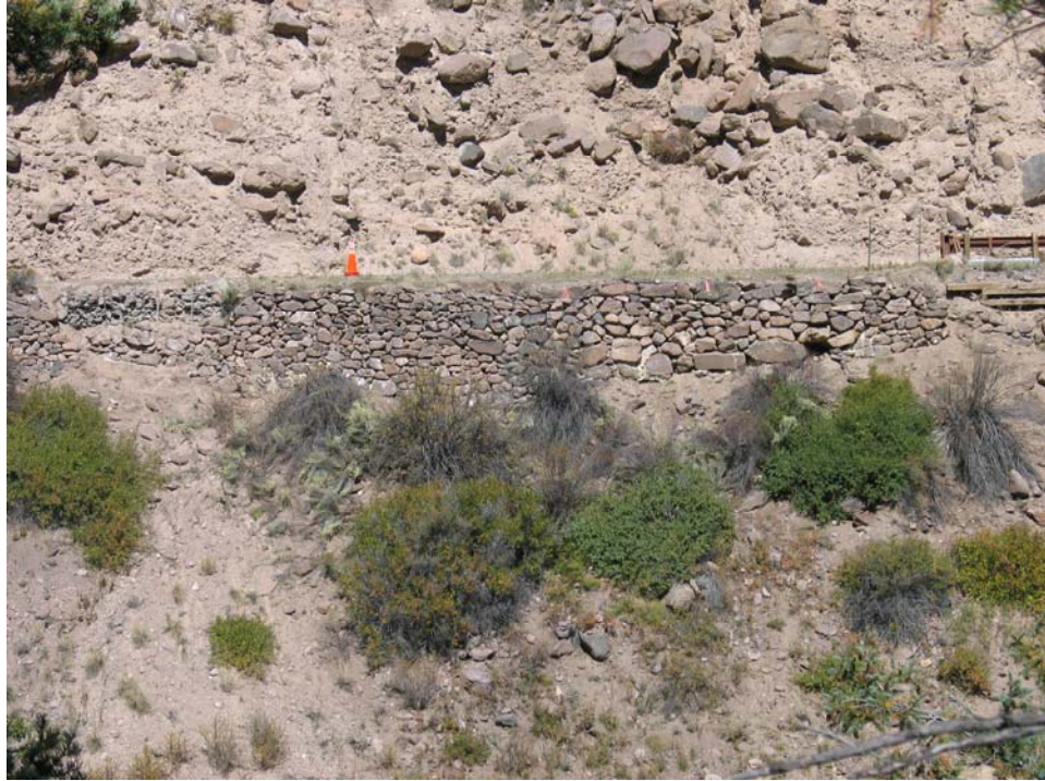
Figure 25. Photo. Elevation view of the South Fork dry-stack wall following completion of PUR injection. PUR overruns are nearly invisible from this distance.
