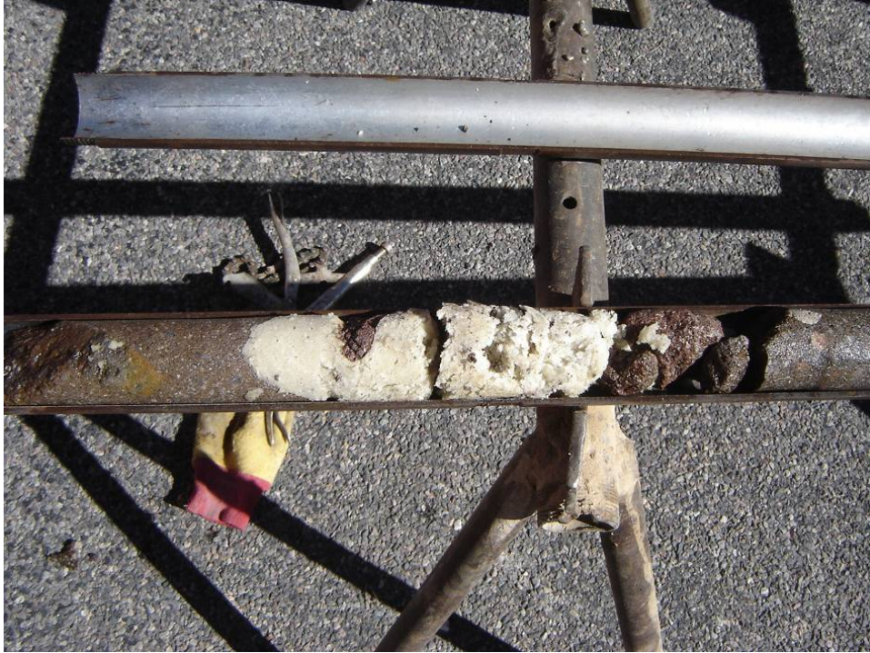
Figure 23. Photo. Light-colored, foamed PUR in core sample.
