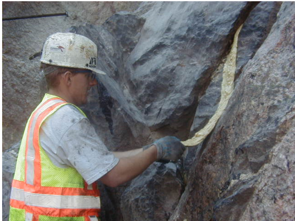
Figure 11. Photo. Rapid removal of expanded PUR product immediately following injection and prior to set. Removal typically requires hand tools following set.
