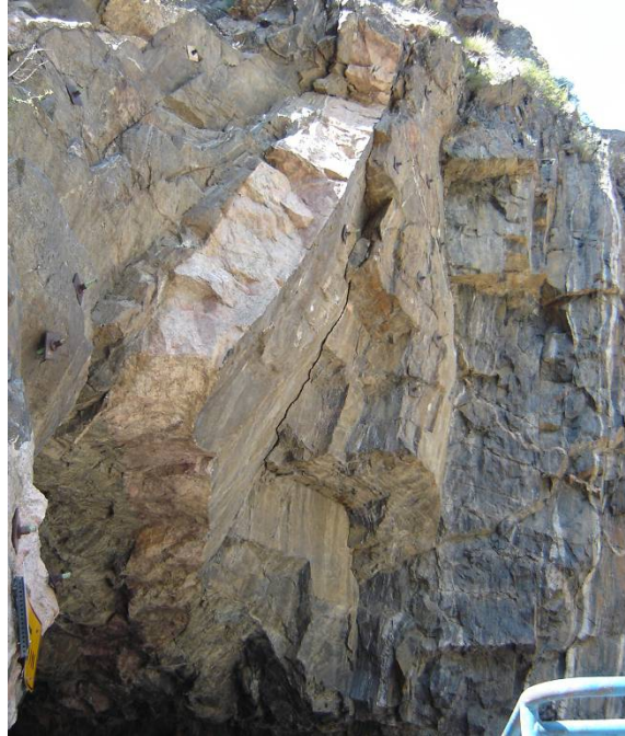
Figure 4. Photo. Close-up of the foliation joint-defined blocks above the western portal and previous spot-bolting.
