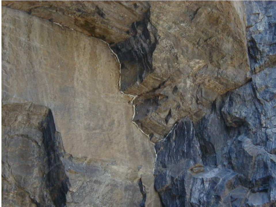
Figure 12. Photo. Single-component PU product used to seal fractures in order to inject PUR product into rock fractures.
