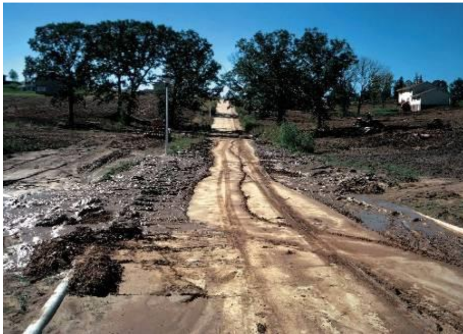
Figure 7D-1.01: Sediment in Street Due to Inadequate Erosion and Sediment Control During Construction
