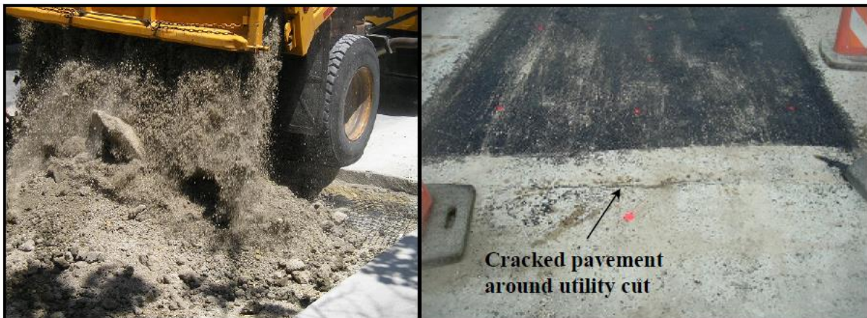
Figure 9D-1.01: Cracking Pavement Surrounding the Utility Cut Area Because of Construction Equipment Getting Too Close to the Edge of the Open Cut
