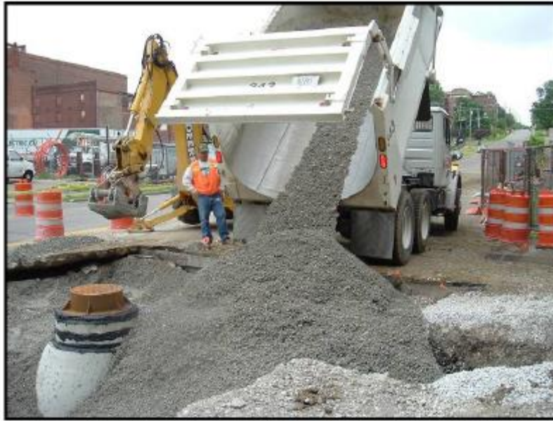
Figure 9D-1.02: Large Lift Thicknesses Used in Utility Cut Trench Backfill Material Placement
