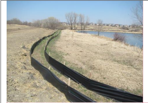
Minnesota Stormwater Manual
