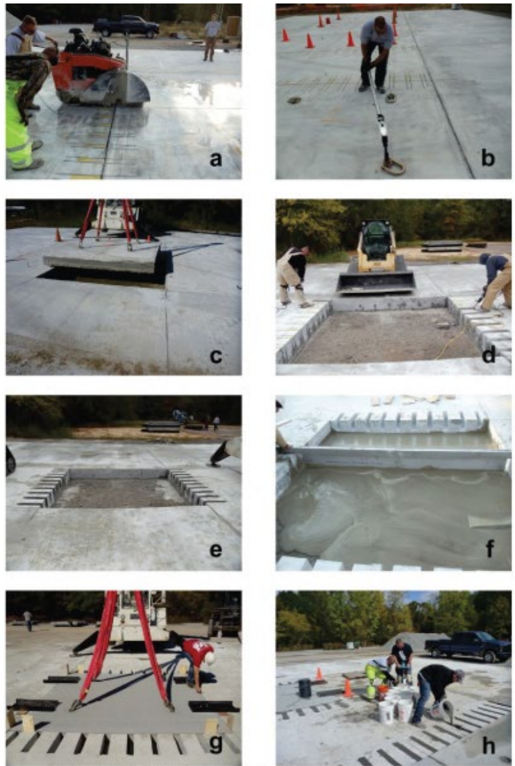
(a) Saw cutting perimeter, (b) installing lifting eyes, (c) lifting pavement, (d) preparing dowel slots, (e) prepared repair area, (f)
