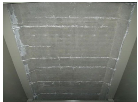
Transverse Cracking on Underside of Bridge Deck
