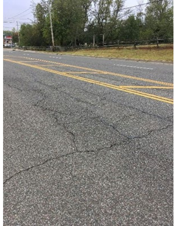
Moderate-severity fatigue cracking in HMA
