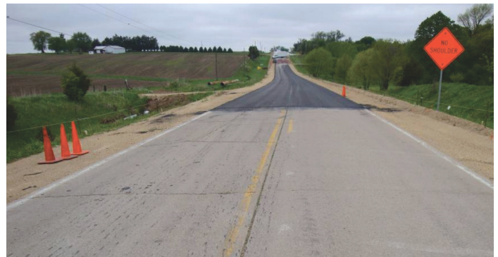
Figure 3. Application of Asphalt Separation Layer to Existing Concrete Pavement for Unbonded Concrete Overlay.
